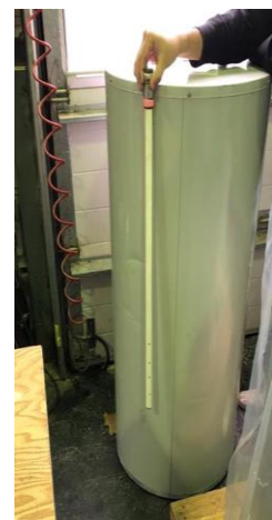
Figure 79: Measuring the Half-height Tank Location
