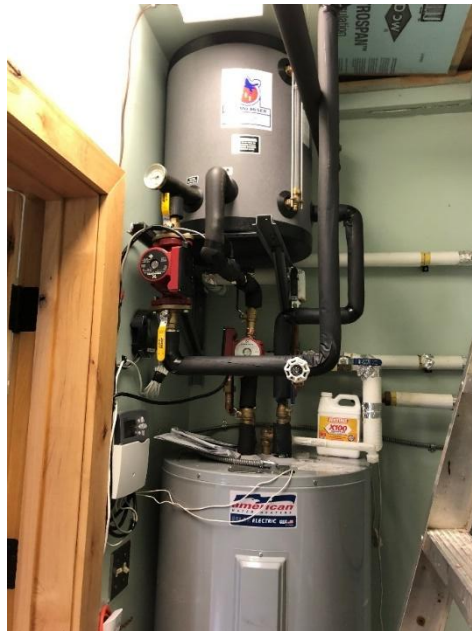
Figure 89: Front view of demonstration installation showing new electric solar storage tank, drainback tank and controller at Missanabie Cree First Nation, May 2022.
