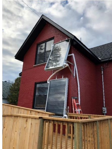
Figure 88: Side view of demonstration installation showing solar thermal collectors at Wahkohtowin Innovation Centre, Chapleau, Ontario, 2021.
