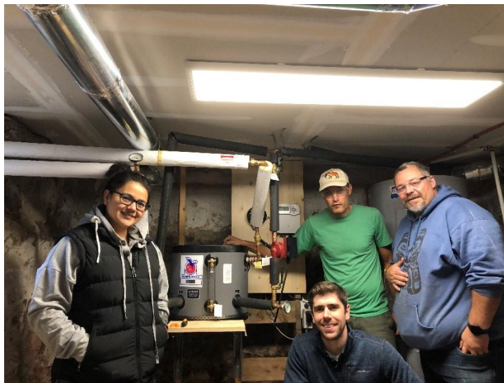
Figure 86: Front view of demonstration installation showing drainback tank, controller and new electric solar storage tank at Wahkohtowin Innovation Centre, Chapleau, Ontario, 2021.
