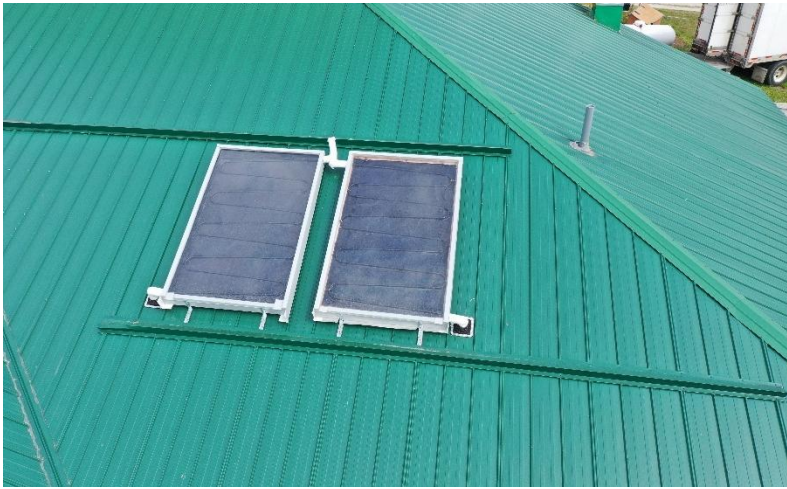
Figure 90: Top view of demonstration installation showing solar thermal collectors at Missanabie Cree First Nation, May 2022.
