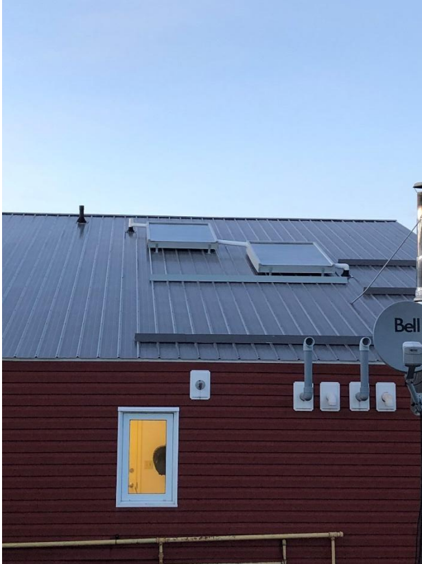
Figure 91: Front view of demonstration installation showing solar thermal collectors at Chapleau Cree First Nation, Mukeso House, September 2022.
