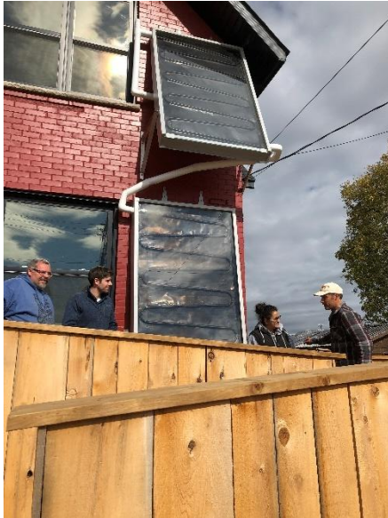
Figure 87: Front view of demonstration installation showing solar thermal collectors at Wahkohtowin Innovation Centre, Chapleau, Ontario, 2021.
