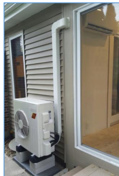
Figure 7: Ductless mini-split ASHP
