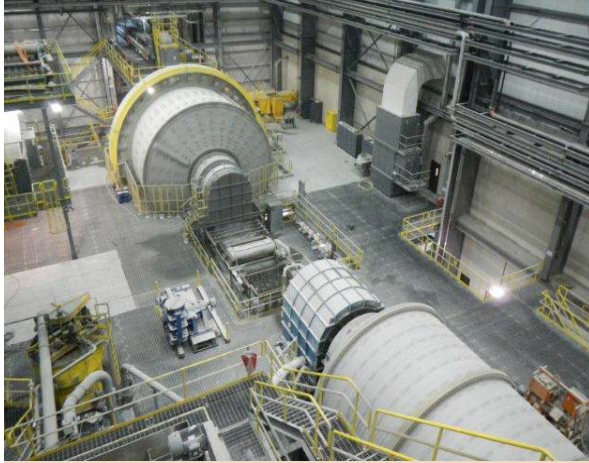
Photo: New Gold Inc. The grinding circuit mills break solid material into smaller pieces.
