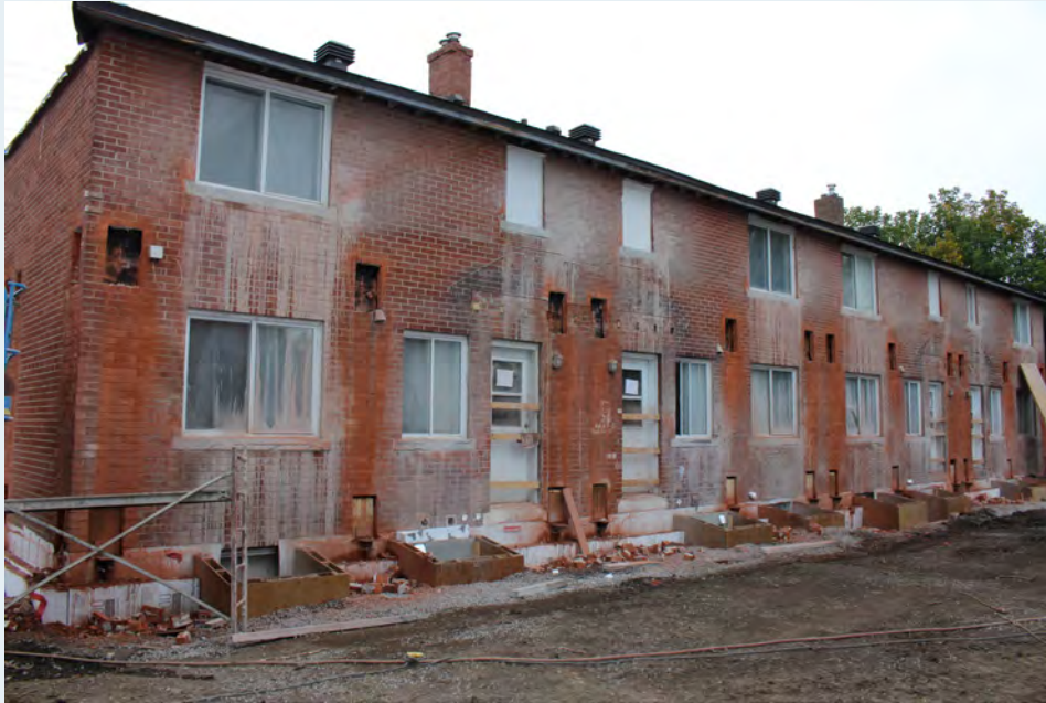
Figure 3-11: Building prep for a PEER retrofit. Canopies, stoops, eaves removed, windows sills cut flush, brick units removed to make structural connections
