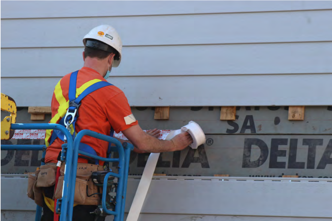
Figure 10-3: Pressure-sensitive acrylic tape being used to seal horizontal panel joint in the field.
