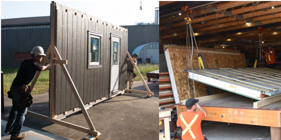
Figure 9-5: (left) Wood outriggers on castors proved to be an affordable and effective way to move panels for the 2017 PEER pilot (right) OCH used hand chain hoists mounted to runners on a steel C-channel that allowed panels to be easily tipped-up and moved within the shop.
