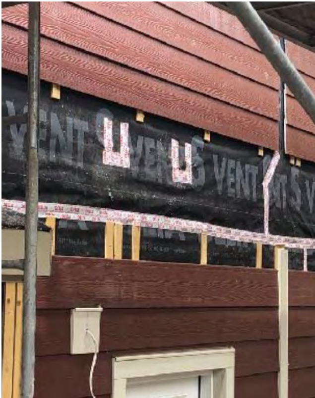
Figure 10-5: Butterwick Projects finished the horizontal panel joints on site by weaving lap siding together from the top and bottom panels together.
